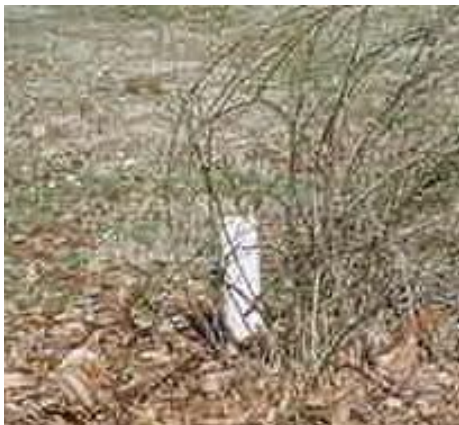
Pump-out Point for Septic system
